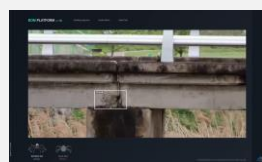
Risk (crack, hole, etc.)
